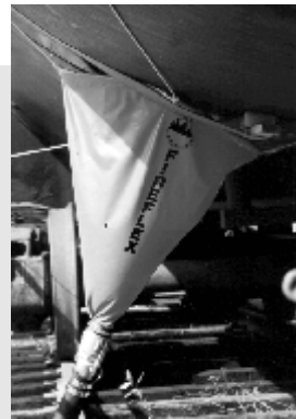
The open end of the Gravity Feed Funnel fits tightly over the leaking area.
